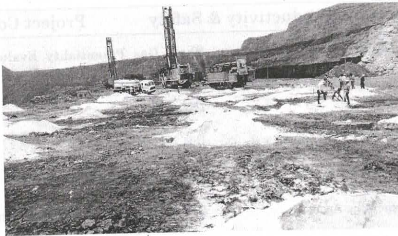
The views of the charging of blast holes at Hard overburden bench of East section of Nigahi Project, Northern Coalfields Limited — MT/164
