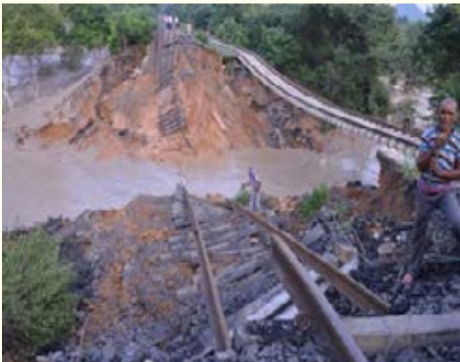
Fig.-10: Damage to Railway track
