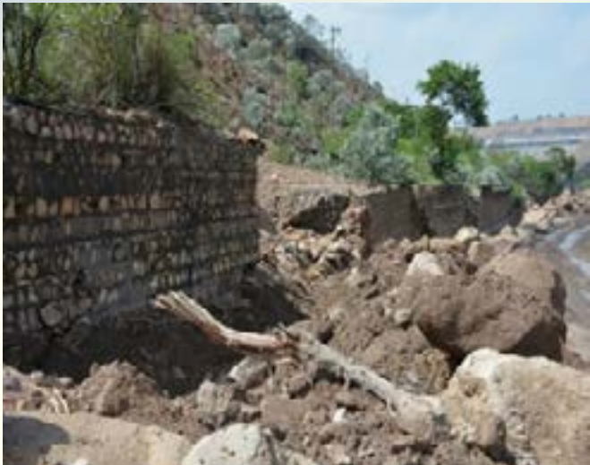
Fig.-9: Damaged RRM Wall
