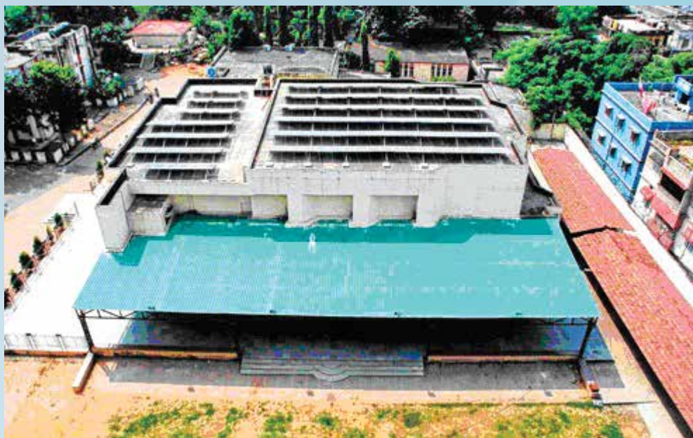
Figure 9 : Roof- top solar power plant over Ravindra Bhawan of CMPDI (HQ) Ranchi.
