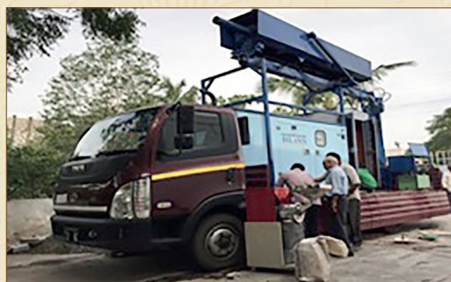
Fig-6: The Hydraulic driven Drilling Mechanism mounted on the truck with other equipment.
