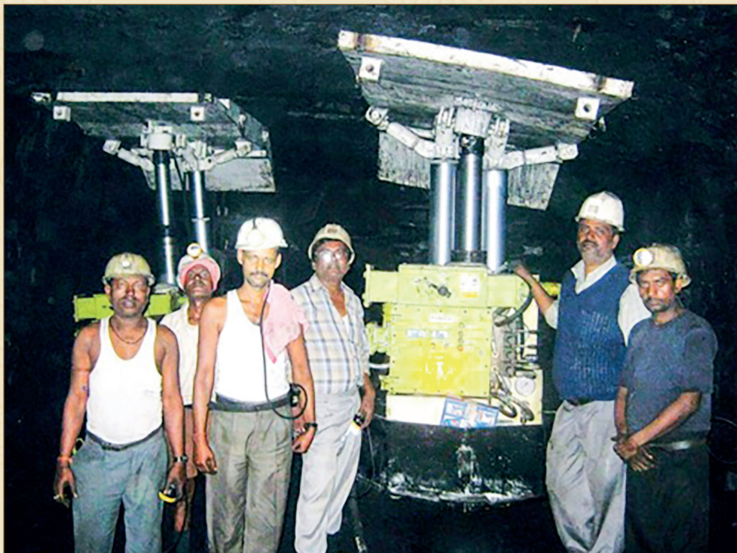
Fig.-3: SAGES at installed at a Goaf Edge in II-D panel, seam no. 2, Victory pit, Bastacola underground mine, BCCL
