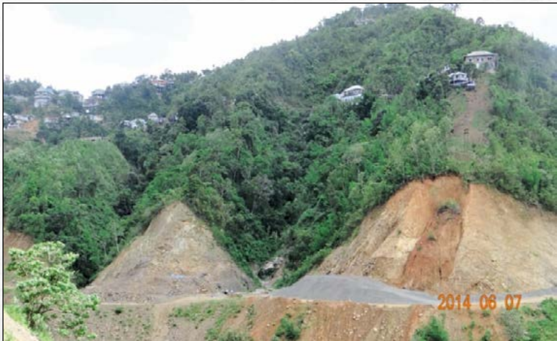
Plate-3: View of rocky portion that required blasting operation at Ch: +2150 m
