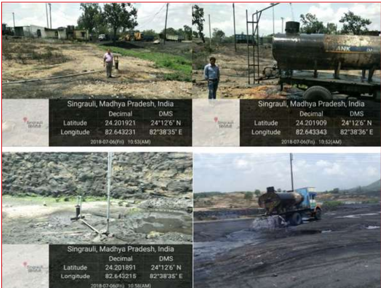
Figure 9: Deep Tube wells (TW1 to TW4) with water filling system for dust suppression by water sprinkler at Morwa Spur Siding
